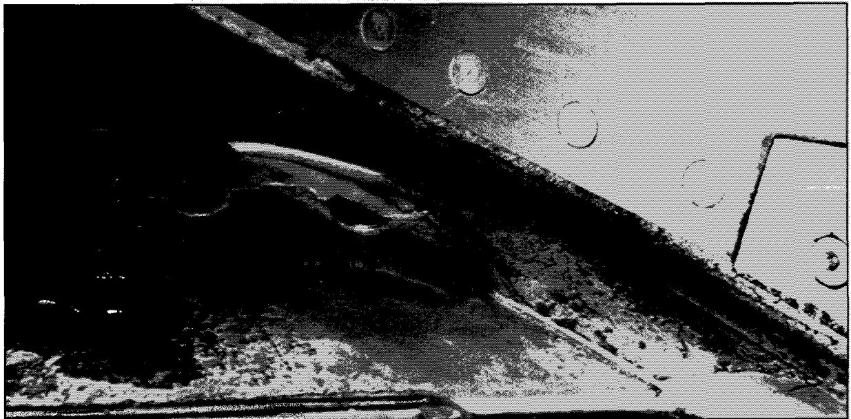
FIGURE 6-7. INCOMPLETE REMOVAL OF CORROSION PRODUCTS RESULTED IN REOCCURRENCE OF CORROSION
