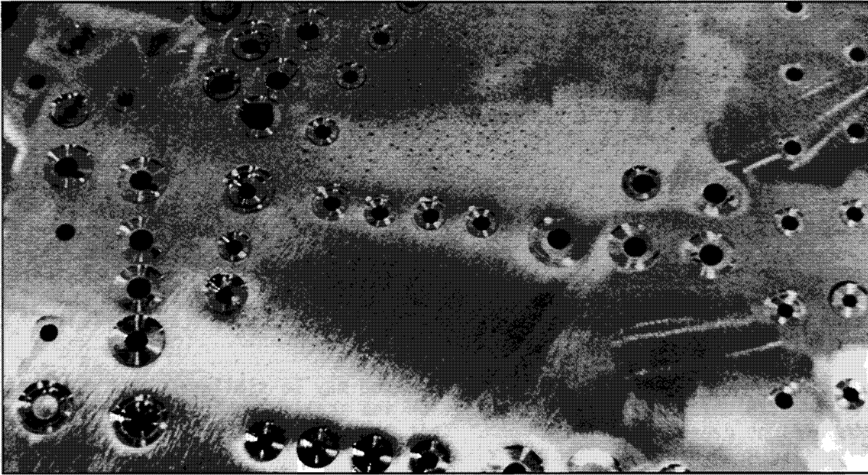
FIGURE 6-9. CORROSION AT FASTENER HOLES REMOVED BY SPOT FACING
