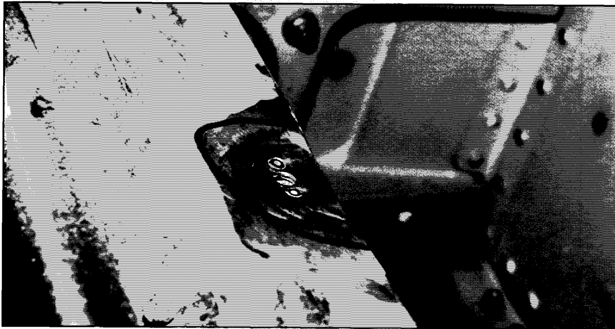
FIGURE 6-5. STEEL PARTICLES FROM FASTENERS OR NUTPLATES MAY CAUSE FUTURE CORROSION PROBLEMS IN ALUMINUM STRUCTURE
